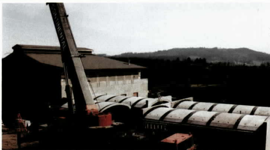
Photo above: Crane lifts vaults into place. Approximately one-half of the vaults have been installed in this photo. Black stripes are sealant used where units come together. Phase I building is at left.
